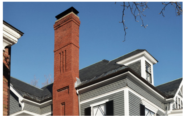
Chimneys with decorative brickwork, such as these inset panels and corbeled coursing, are distinctive and should be preserved.
