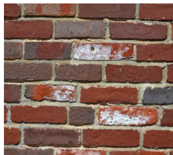
Efflorescence is a white haze caused by the migration of salts through masonry units.
