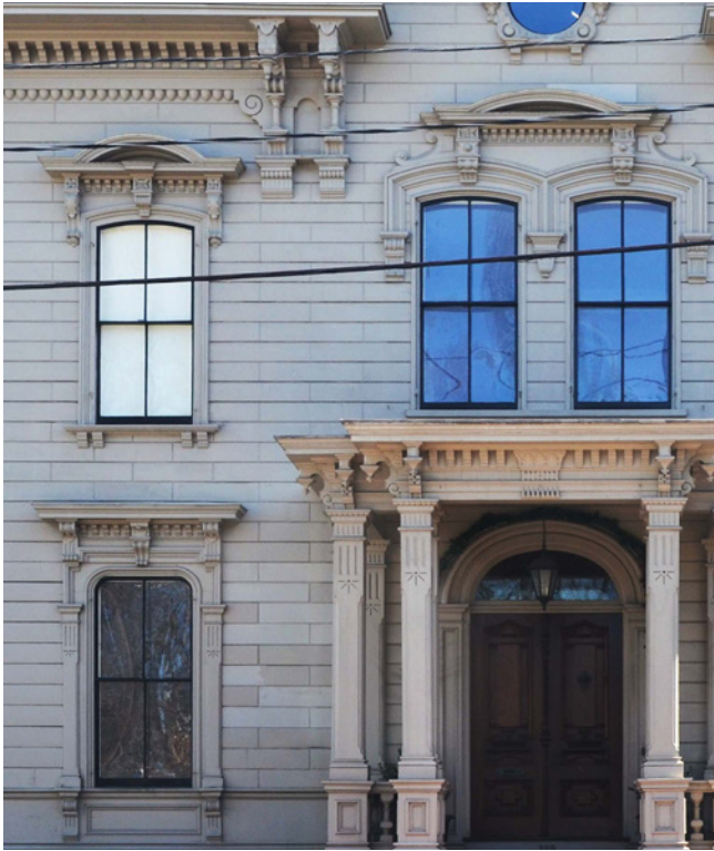
Wood siding and richly detailed wood trim should be preserved. Rusticated boards were historically used to imitate masonry.
