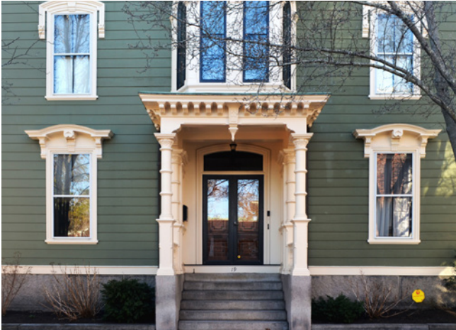
Ornate Second Empire and Italianate columned entry, carved wood double doors (behind storm doors), and a segmental arch transom.
