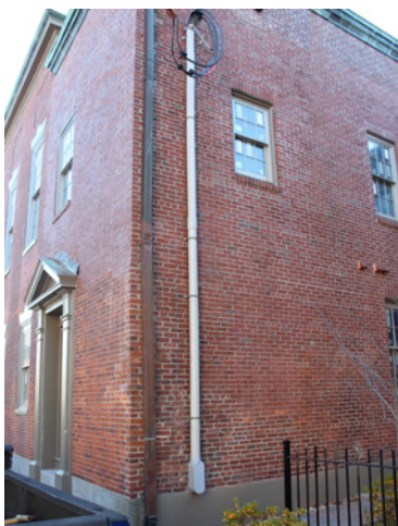
Communications and electricity wiring can be consolidated and strung to a single point. Locate wiring at secondary facades and building corners to minimize visual impact.
