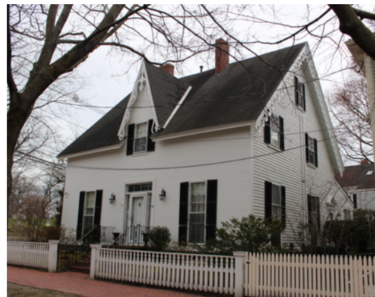
An example of well-preserved wood flushboard siding, clapboards, and gable-end vergeboard trim.
