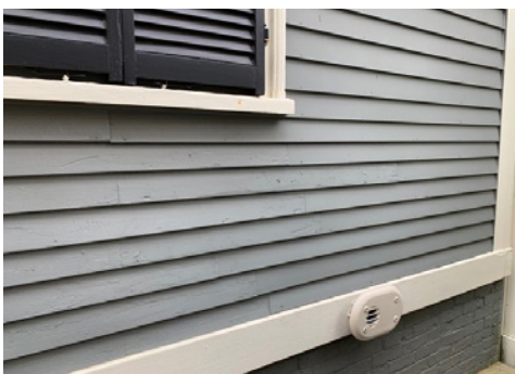
A mechanical vent located on a skirtboard and painted to match is an appropriate installation.
