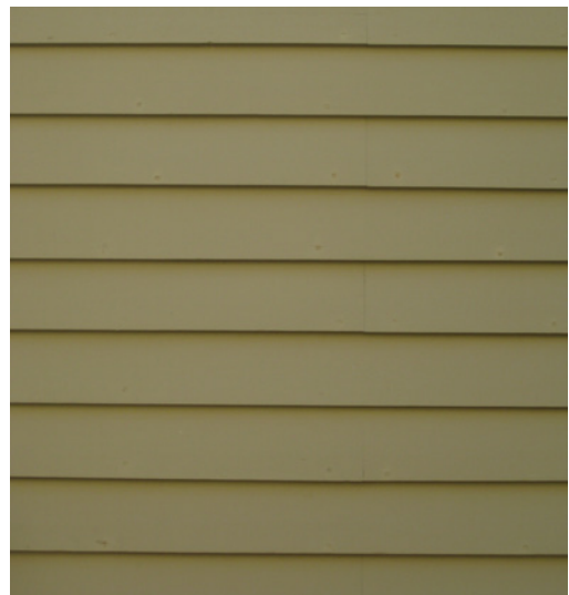
Painted wood siding is the most historically appropriate material. Siding with the wood grain side facing out or faux wood texture is not appropriate.
